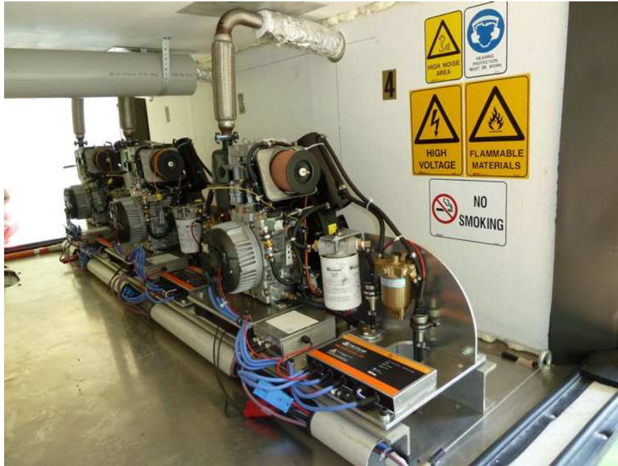
Figure 3. Inside the PLATO-F Engine Module, showing three of the five diesel engines. A fuel bladder, containing 6000 litres of Jet-A1, is immediately below the aluminium plate at the bottom of the figure.
